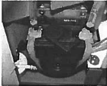
Pump with loosened tubing holder.
