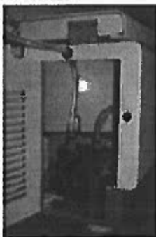
Access door open with pump visible.
