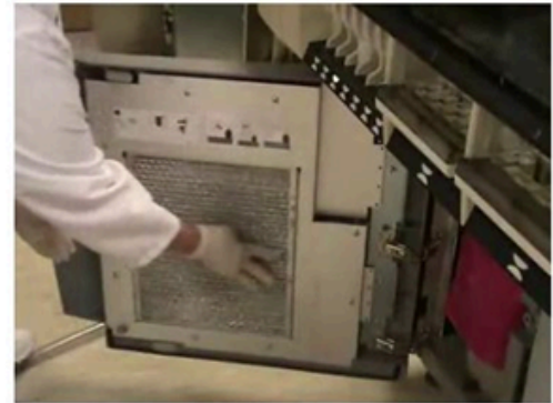
Clean Air Filter #2
