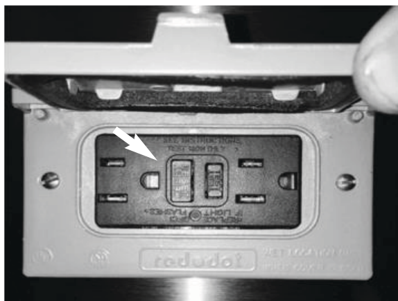
Figure 4-2. Reset Button on GFCI Outlet
