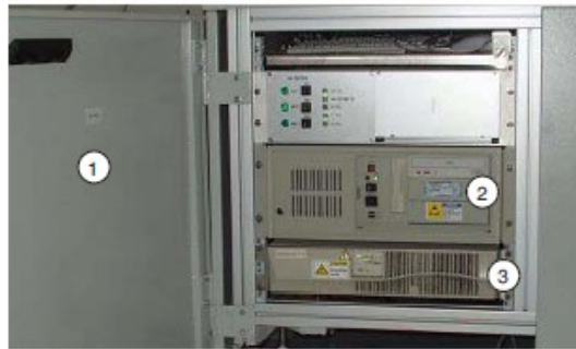
1. Input/Output module front-left door 2. Computer 3. UPS
