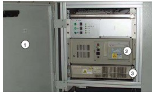
Figure 5.1: Input/Output module computer/UPS storage center
