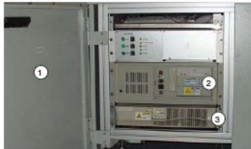
Figure 5.16: Input/Output module computer/UPS storage center
