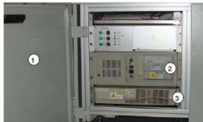
Figure 5.7: Input/Output module computer/UPS storage center
